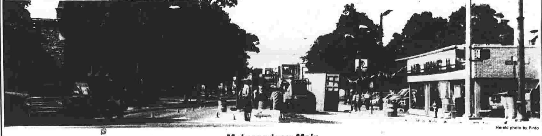
Construction crews begin installing a new sewer main on Main Street Tuesday as part of the $1.6 million Porter Street sewer project. The Main Street portion of the project will be the most expensive and time-consuming. Water and Sewer Administrator Robert Young has said. The Glenn Construction Corp. of Manchester has already finished work along Hill, East Center and Porter streets.
